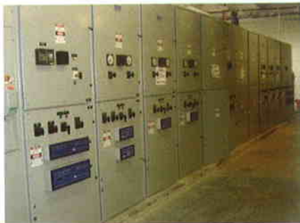
Primary switchgear in the Diamond Head electrical room; Kiewit Building Group completed the project.
