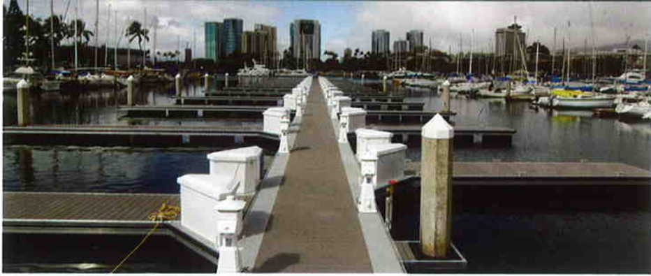
The newly completed floating docks for Dock "B" at the Ala Wai Small Boat Harbor by Hawaiian Dredging Construction Co., Inc. The $2.8 million contract included replacing the existing floating and fixed docks with new floating docks and utility systems. Approximately 140 boat slips will be upgraded in time for the 2009 Transpac.
