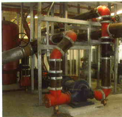
Chilled water and condenser water pumps and piping in the new Diamond Head chiller plant built by Kiewit
