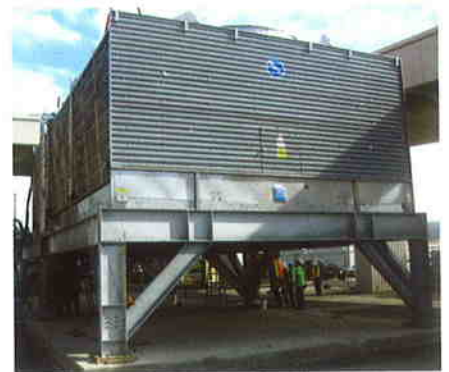
The new Diamond Head air-conditioning chiller plant at Honolulu International Airport is 50 percent more energy efficient and has a greatly increased load capacity than the former facility.
