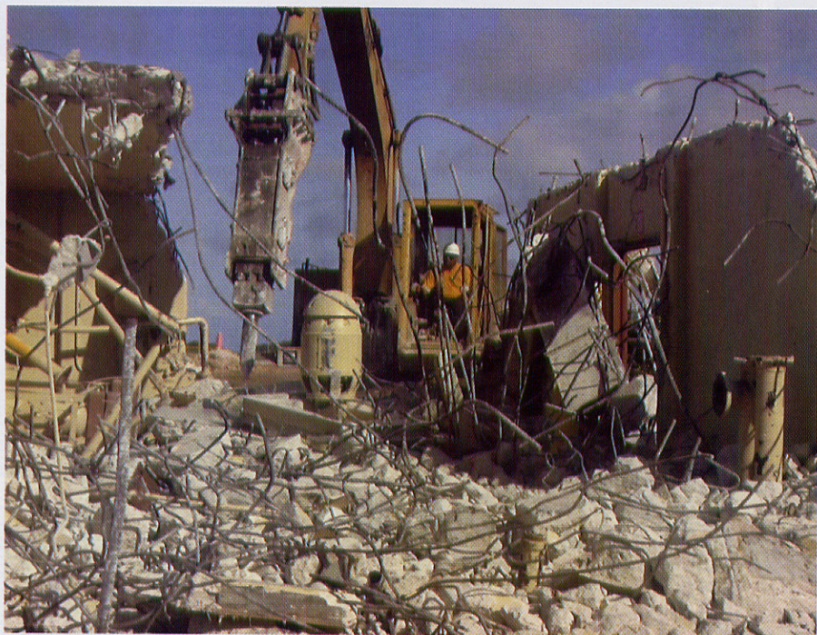
As part of Phase II of Andersen Air Force Base's POL Hydrant Fueling System and Consolidated Fuels Project, 10 inoperative fueling pits and two pump houses were removed by Nova Group Inc. Nova is scheduled to complete Phases V and II of the five-phase project in October.
