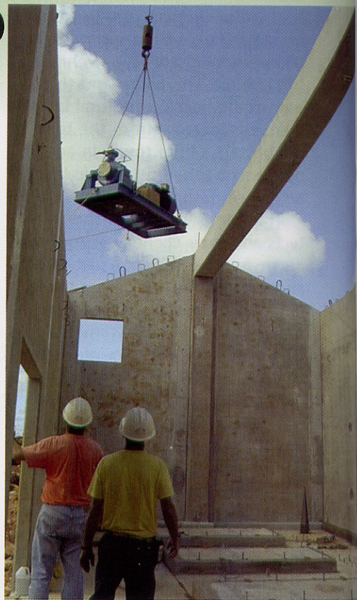
A pump is lowered into a facility as part of Phase V of Andersen Air Force Base's POL Hydrant Fueling System and Consolidated Fuels Project.
